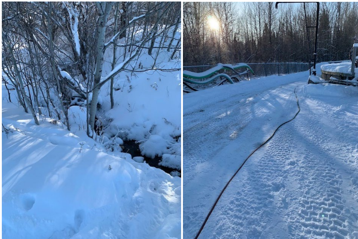
Photos 1A (left) & 1B (right): New dechlorination contact chamber outfall area & general area where new pipe tie-ins will be required to connect clarifier outlets (partial view can be pictured right) to new dechlorination contact chamber
