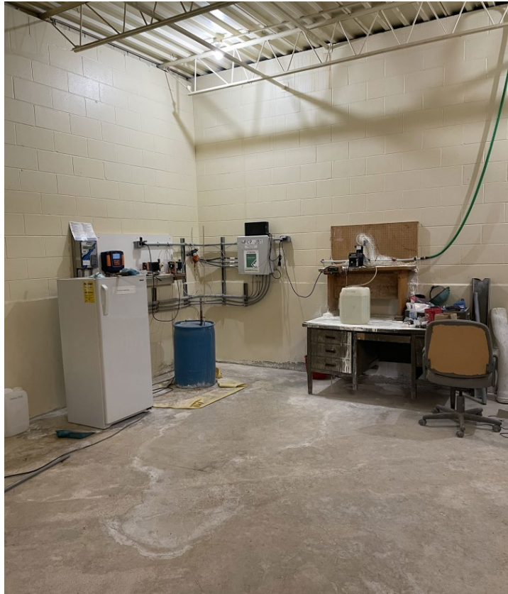
Photo 1: Service Building Interior (Chlorine Dosing System)
