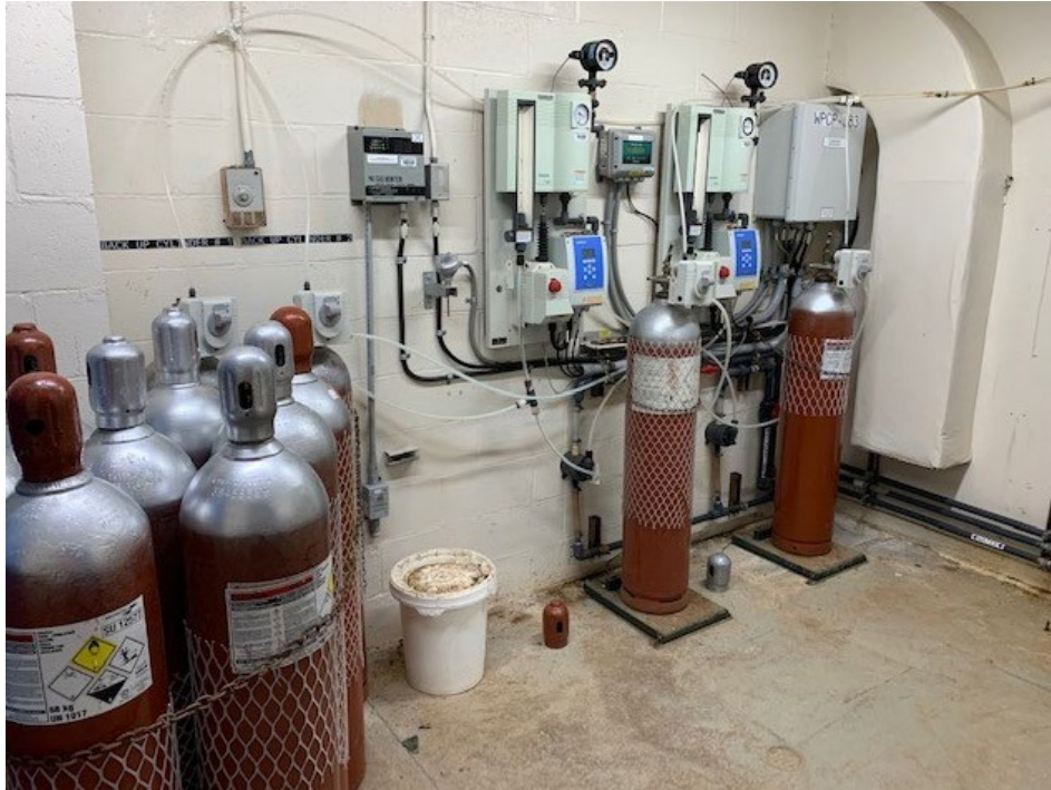
Photo 2: Interior of Service Building (Chlorination Dosing System)
