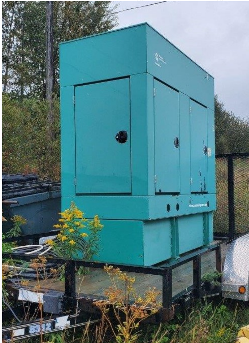
GRNPSLL-015 Cummins Generator & Trailer
