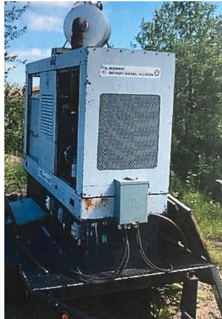
GRNPSGN-016 Saturn Detroit Diesel Generator & Trailer
